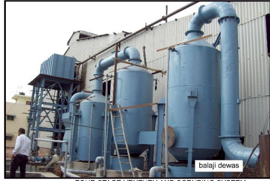
FOUR STAGE VENTURY AND SCRUBING SYSTEM
