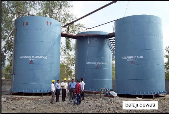
ACID STORAGE TANK
