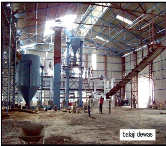
FULL VIEW OF S.S.P PLANT
