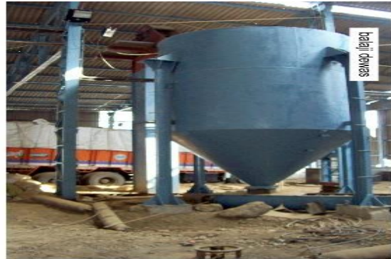
ROCK STORAGE TANK
